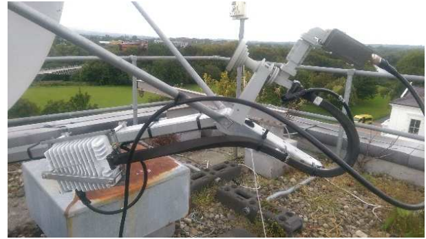
Figure 1. UL Ku/Ku Antenna Equipment.
