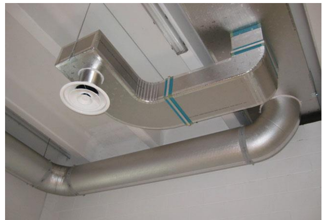
Figure 1. Example of circular and rectangular metal structures used as ventilation pipes.
