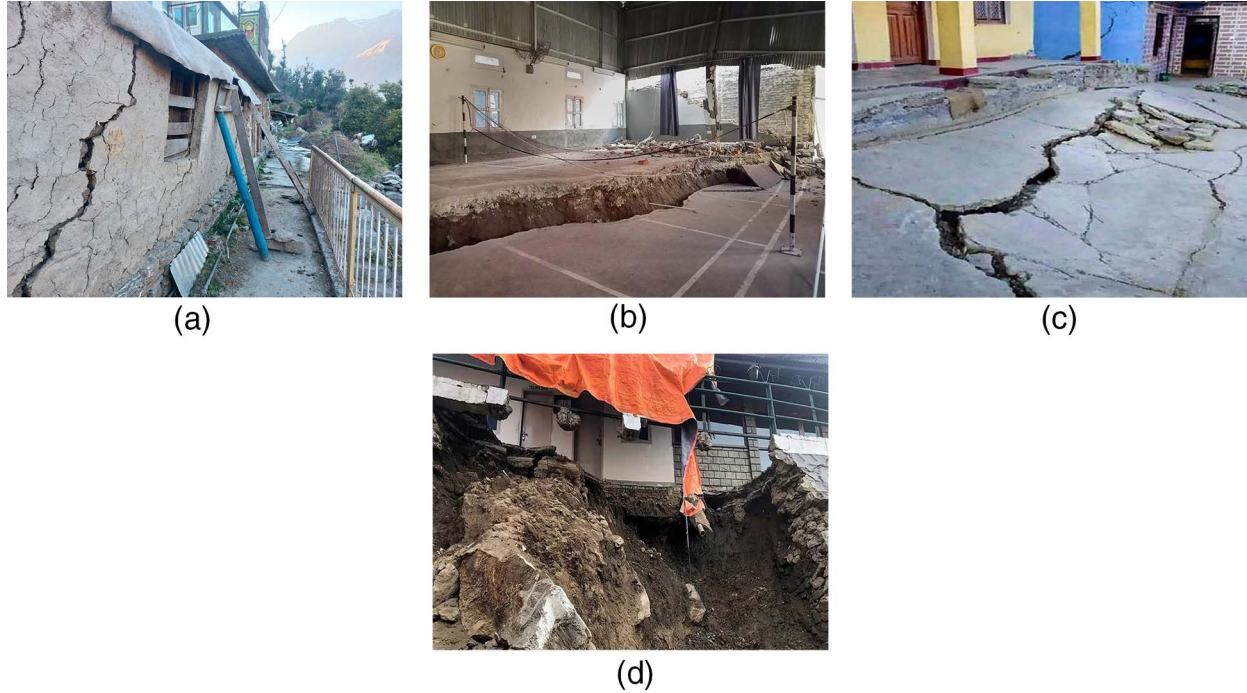
Figure 1. On-site imagery taken from print media. (a) The initial warning from Joshimath was captured by Vajiram and Ravi. (b) Land subsidence in Joshimath, as taken by The Hindu. (c) Some remote areas were affected by the talks with ISRO. (d) Impact on 65% of the houses recorded by the government.
