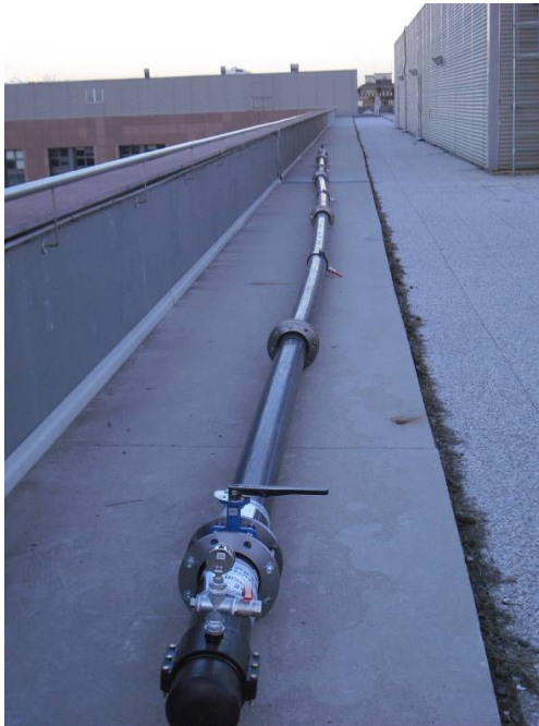
Fig. 1 The test set installed on the roof of Politecnico di Torino
