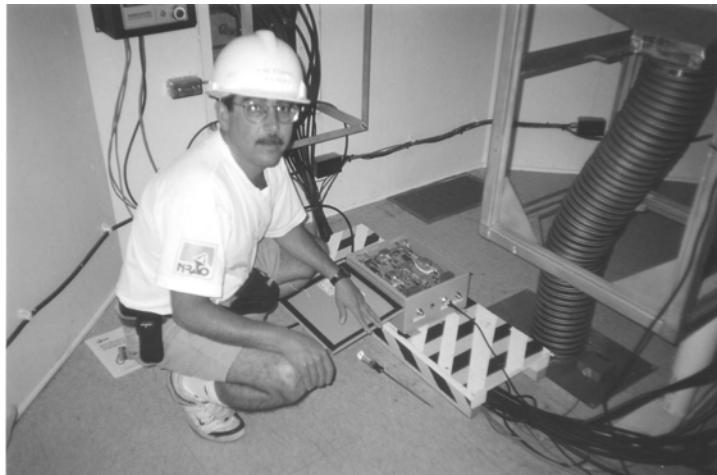
Figure 2. 74 MHz receiver being installed in VLBA-Pt vertex room.
