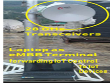
Figure 7: 5G Mobile Gateway on Mobile trolley
